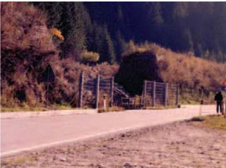
Figure 32 - The great reinforced earth wall which partially protects the road from the rocks falling from the lower parts of the Ruinon slope.
