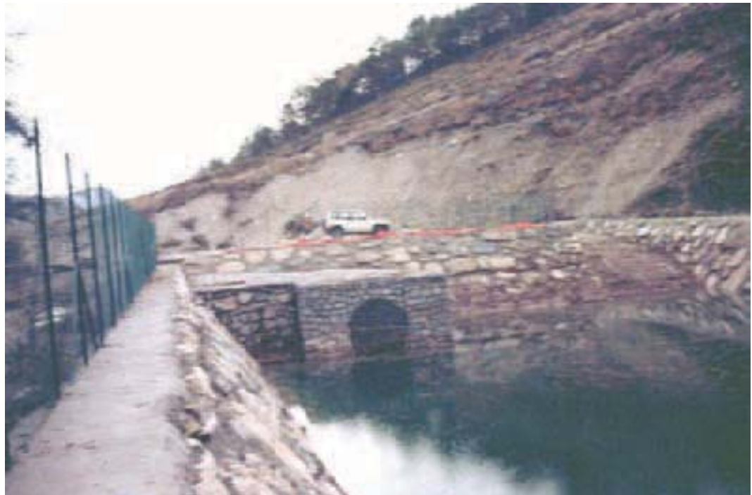
Figure 68 - The intake construction built after the event to allow a safe remedial work realization. The work is located at the left edge of the accumulation body, which has dammed the river bed. The water are collected from the Magnone stream and discharged downstream to avoid the erosion of the landslide foot.
