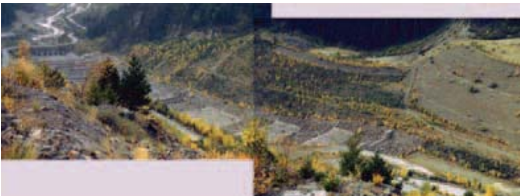
Figure 29 - The repairing works at the foot of the Valpola landslide. On the right it is possible to see the huge earth wall built to protect the new Adda river bed, completely running into concrete walls.
