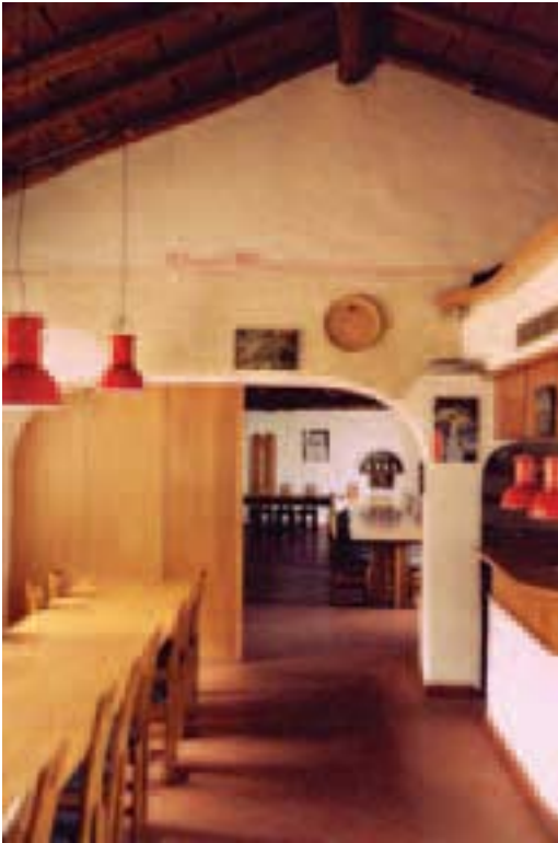
Figure 20 - High-water mark recorded on an inside wall of the “La Brace” bar-and-restaurant at km. 24 of SS 38, left on the buildings by the floodwaters of 17-19 July 1987.
