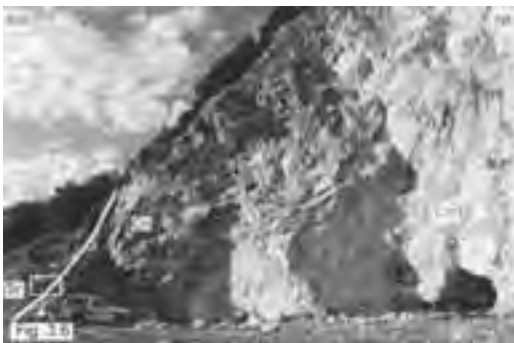
Figure 3.5 - Normal fault separating the Scaglia Rossa Fm. (Sr) from the Calcari Nodulari (Cn). CM: Calcare Massiccio.
