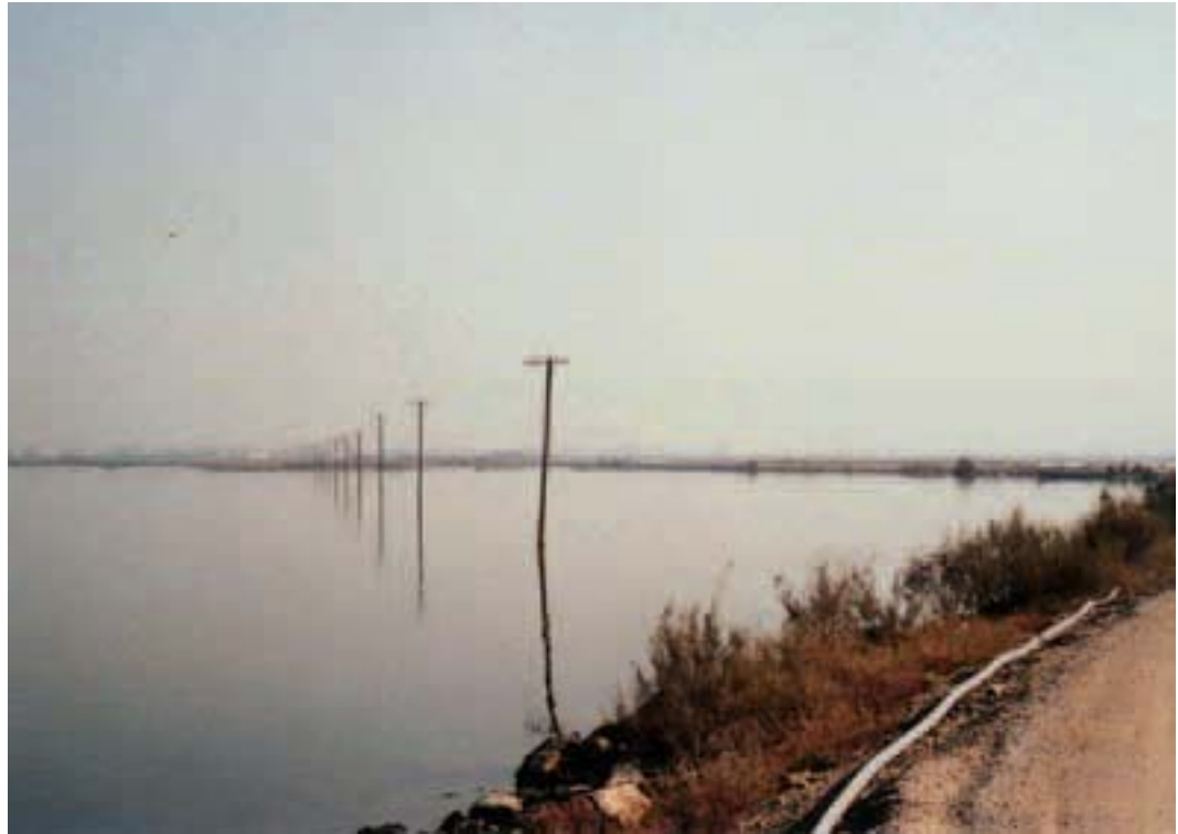
Photo 5.12 - The subsidence is well obvious from the fact that the old road lies beneath the water surface, as it can be seen along the telephone line poles. This happened due to the intensive water groundwater pumping, soil subsidence has occurred and embankments were constructed to prevent seawater intrusion. 8 years ago, one of the dams broke and the sea flooded a large part of the area.
