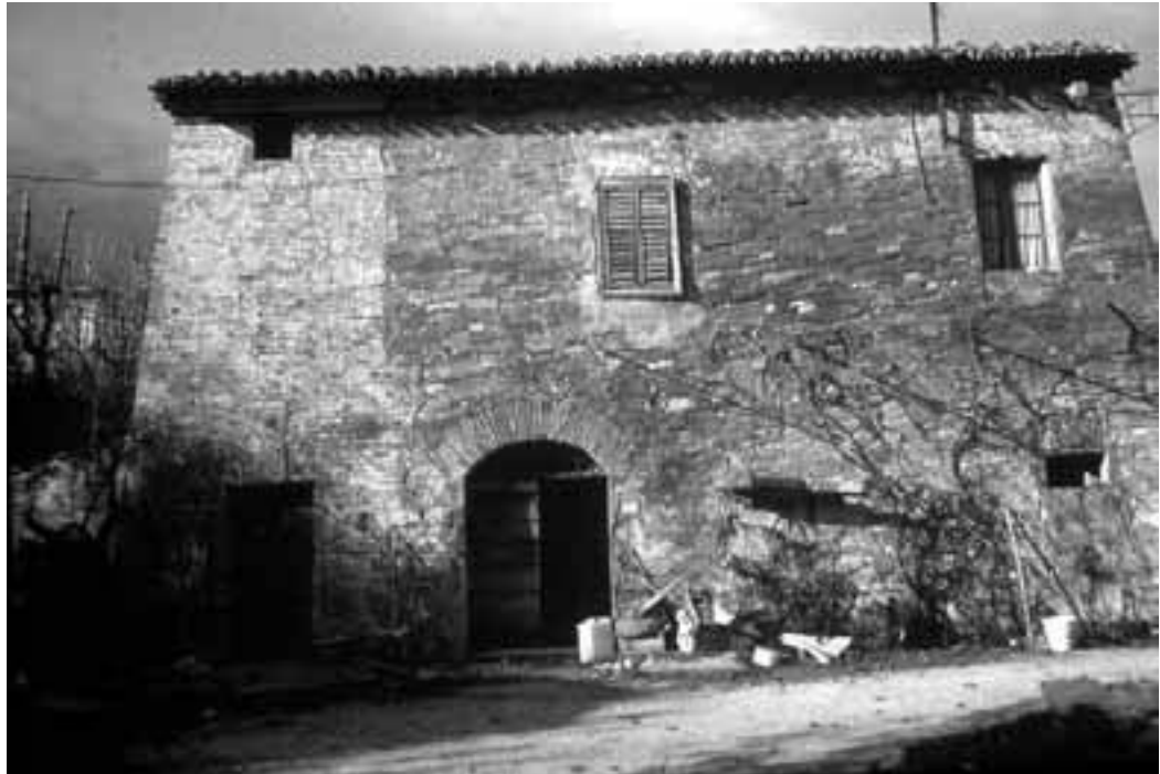
Figure 5.11 - A 16 th century post-house, showing the cumulative effects of recurrent landslide movements on the Montagnolo slope.
