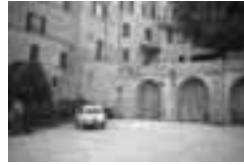
Figure 5.3 - Rupture in the wall which crosses the Montelparo trench. The buildings on the left side are located in the stable portion of the hill; the rupture indicates the upper margin of the trench.
