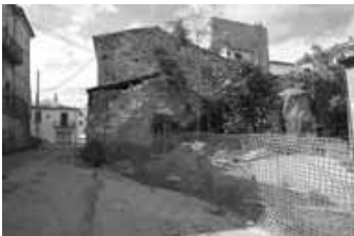
Figure 2.6 - Damage along a reactivated scarplet.
