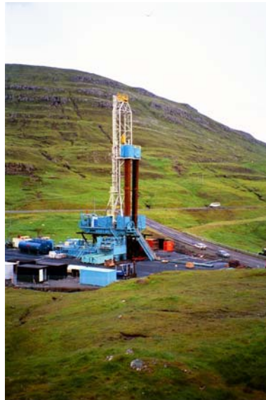
Fig. 78. Drilling rig for the deepening of the Lopra-1 borehole in 1996. Photo courtesy of Turid Madsen.
