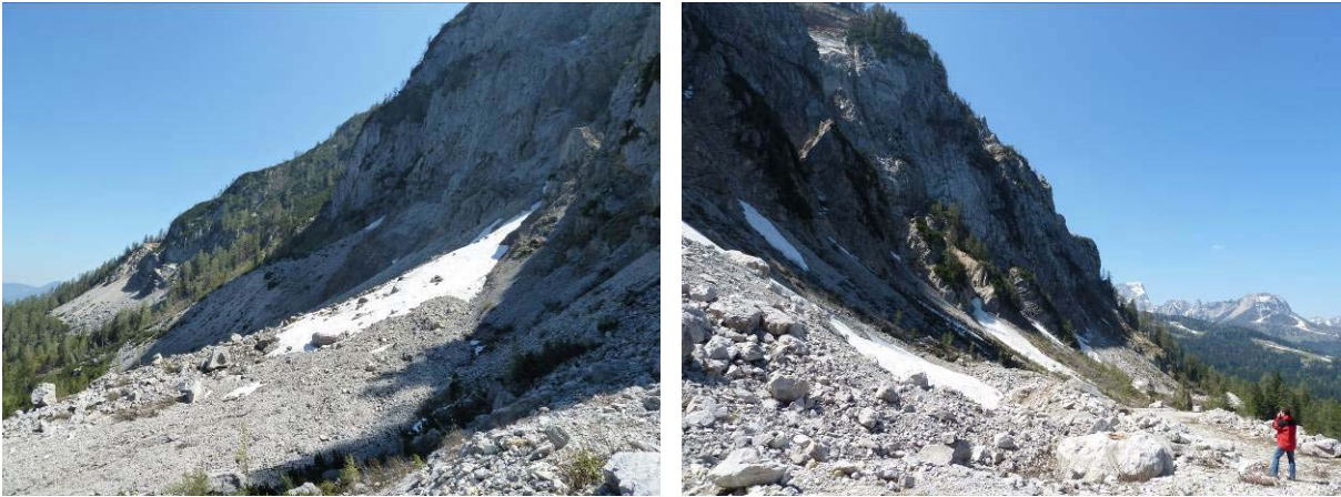
Figure 14. Foot of the rock face of Reppwand (left photo view to the East, right photo view to the West; location 3 in Fig. 1), which indicates the main scarp of the landslide. Rock fall, topple and rock spread processes are evident.
