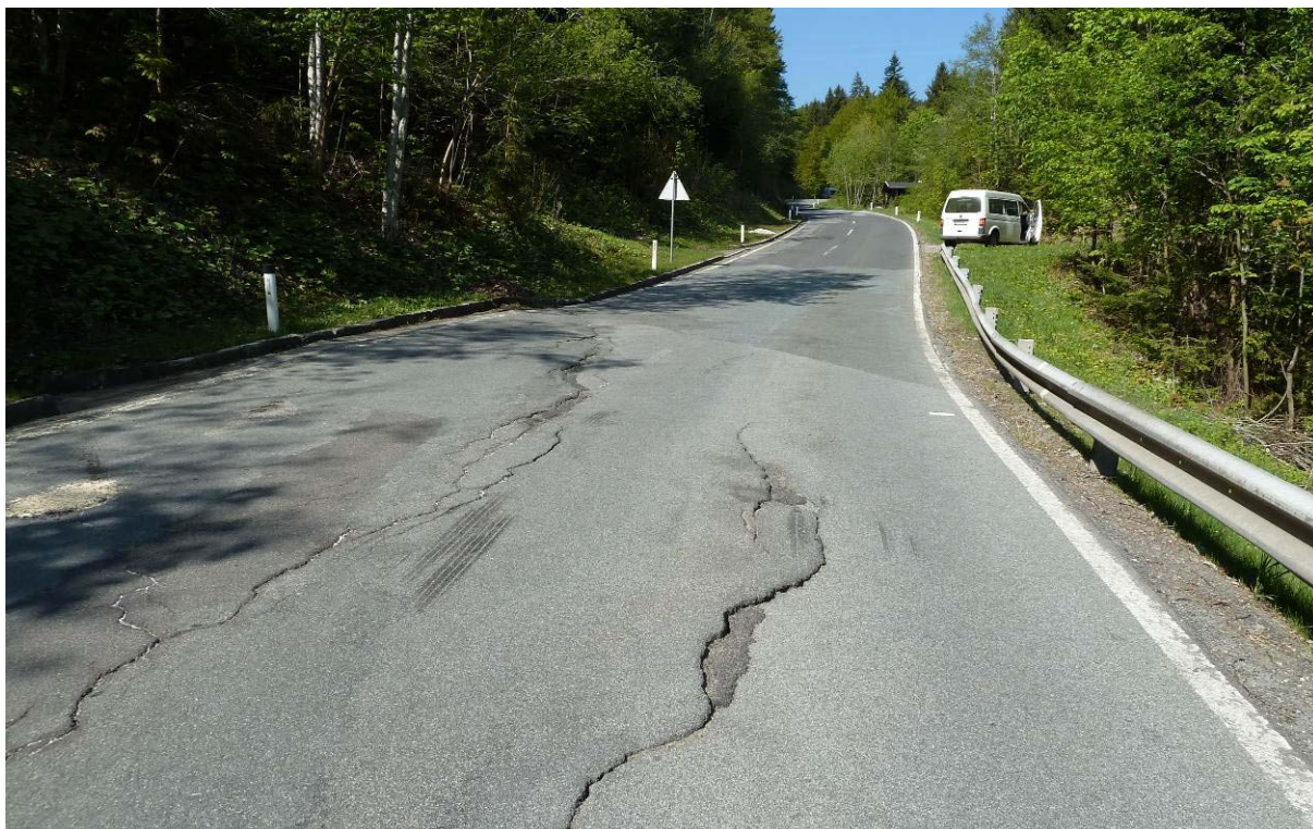
Figure 7. Damage of the Naßfeld road (May 2011) where it crosses the most kinematic active section at the toe of the Reppwand landslide. Average velocities of horizontal displacement of more than 7 cm/a have been detected between 1991 and 2006 (see also Fig. 10).
