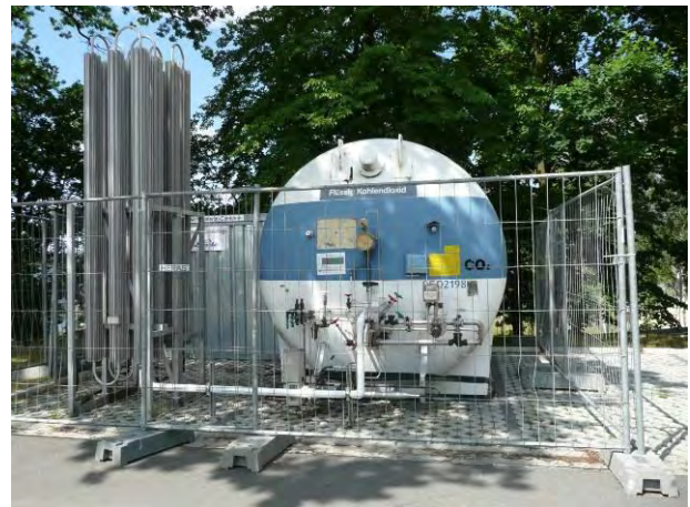
Figure 21: Tank of liquid CO 2 (provided by Linde), Heat exchanger based vaporizer. The gas was transported from the shore to the platform at a pressure of 8 – 9 bar.
