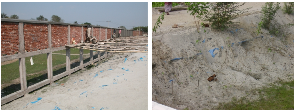
Figure 18 Base foundations in Bangladesh, here at the Titas hospital complex and its access road, consist of alternating layers of sandy material and plastic sheeting (the left picture showing the wall around the hospital complex, was photographed by B. Planer-Friedrich in February '07, the right one shows the access road to the hospital, taken by the author in November '07)
