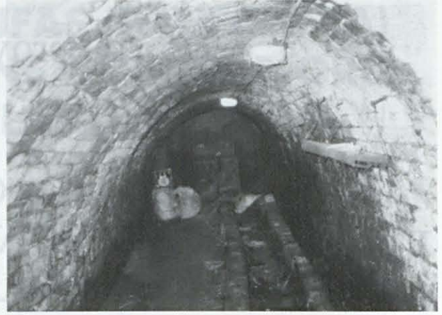
Fig. 4. A strongly deformed cellar tunnel in loess under road No. 56. Dunaszekcső, Baranya county.
