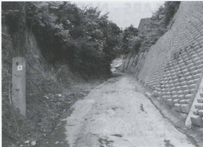
Fig. 1. Typical incised road in loess and a way of slope stabilization, Pécs, Baranya county, Hegyhát balk.
