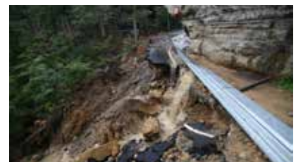
Figure 9: Landslide at the "Preacher's Chair".
