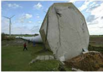
Figure 6: Example of a toppled wind turbine (Nova Scotia Power's Nuttby Mountain) https://ontario-wind-resistance.org/2011/02/03/nearly-all-22-turbine-foundations-cracked/ .
