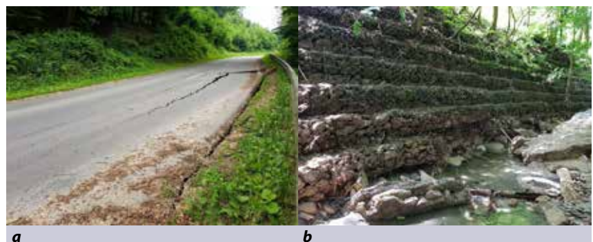
Figure 3: Examples of damage: cracks on the road (a); damaged gabion retaining wall (b).
