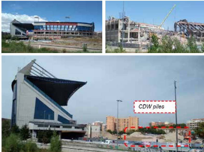
Figure 8: Demolition of Atletico de Madrid Stadium and CDW pile waiting to be re-used (Credit: Pedro Juan García Guzmán).
