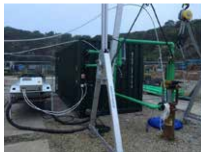
Figure 6: 400 kW Thermal Response Test (TRT) rig with "air blaster" – external and internal viewpoints.
