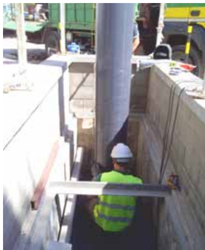
Figure 4: Installation of a suction flow control device (SFCDD) in a water well.
