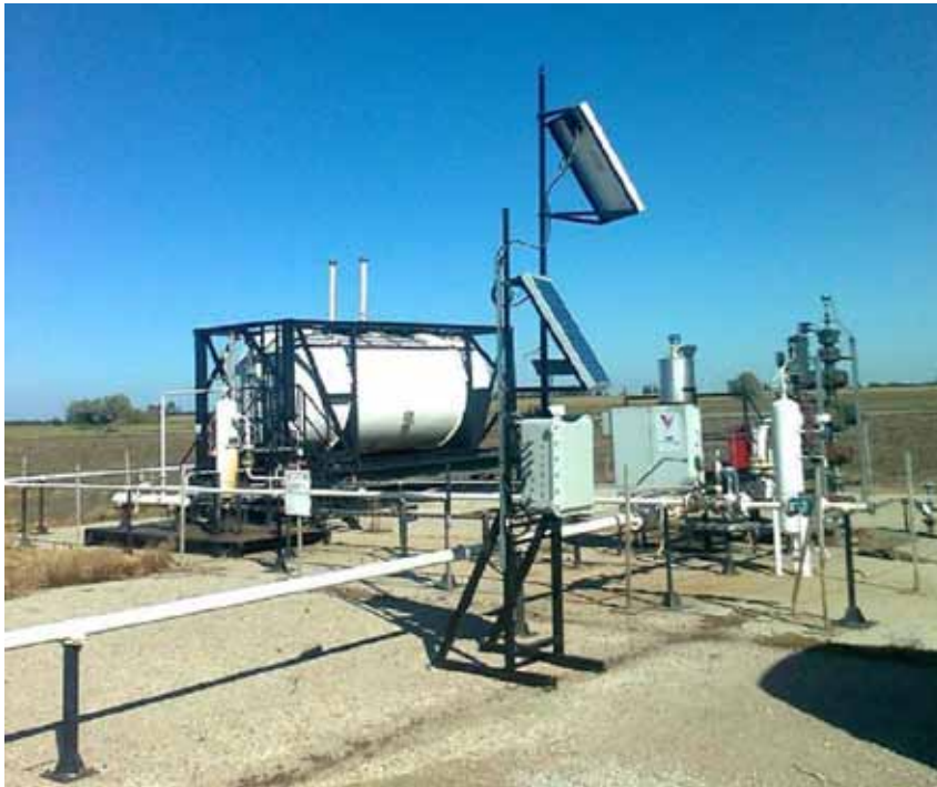
Figure 4: Solar battery-powered mobile communication unit on the wellsite.
