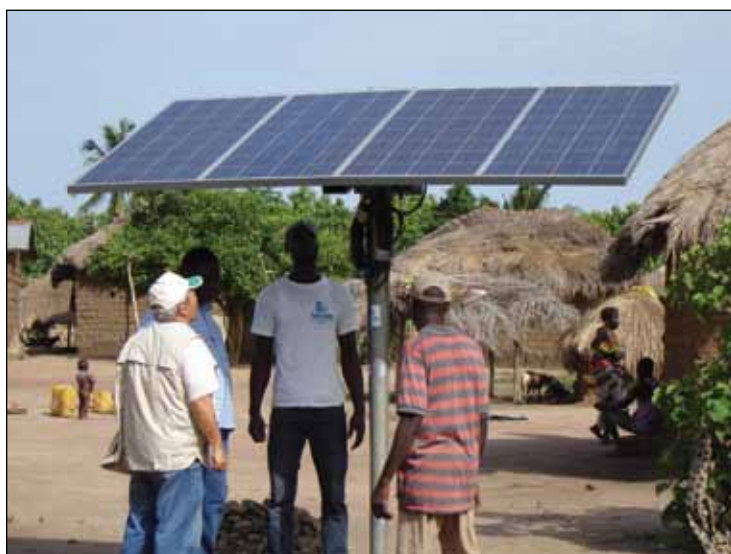
Solar panels for the submersible pump installed in the Avovo village water well
