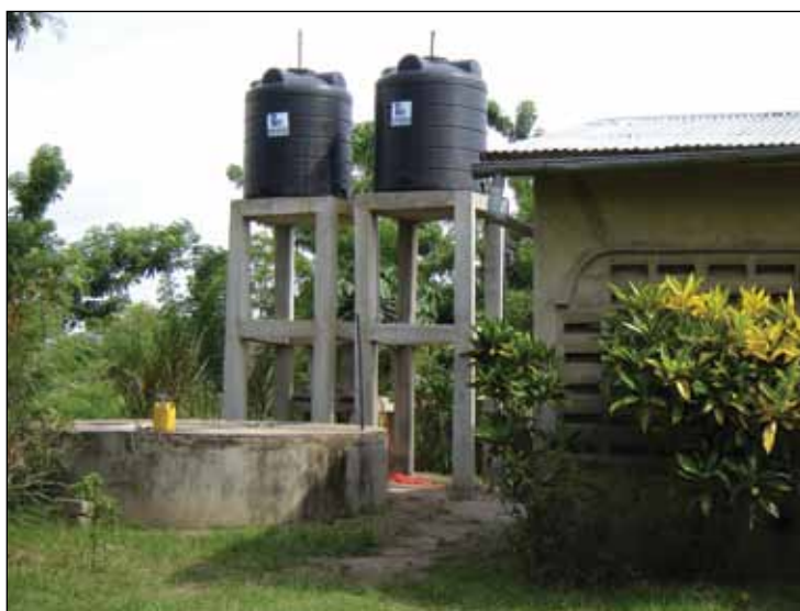
Water distribution system in Fadakope
