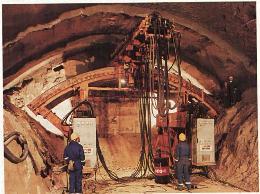
Mechanical precut machine. Roof arch execution Tunnels under El Pardo mountain. Madrid. (Spain).
