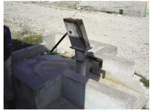
An existing water well in one of the communities included in the project, with hand pump, now completely dry, closed and out of use
