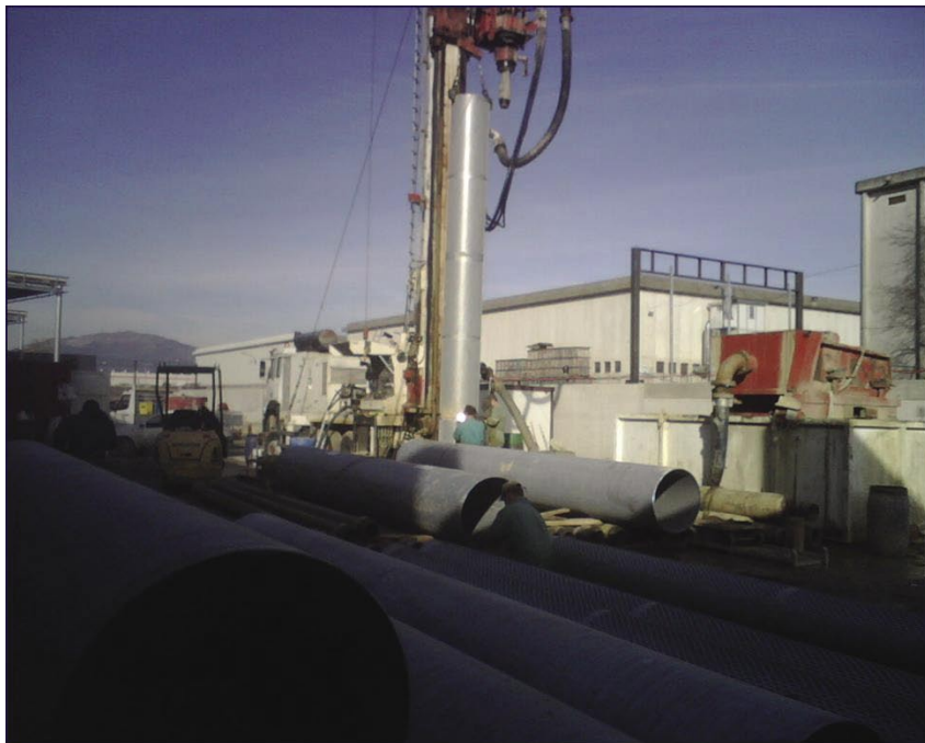
Bergamo (Lombardy): drilling borehole to serve an open loop system by a large commercial mall (total heat power installed over 5 MWth).
