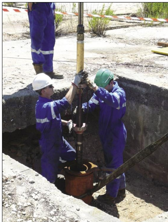
Figure 6. Detailed logging on geomadrid 1 (Cantoblanco project) July 2008 to check well integrity
