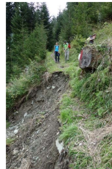
Figure 1: Landslide damage on a hiking trail in the Großarl Valley, Salzburg, Austria
