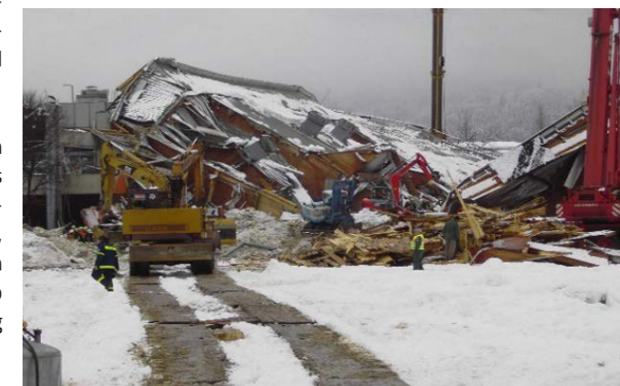
Figure 2. Collapsed roof due to heavy snow fall (photo by Norbert Gebbeken)
