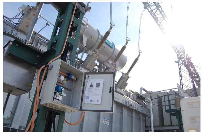
Figure 2: Installed transformer neutral point current measurement system and self-engineered measurement electronic.
