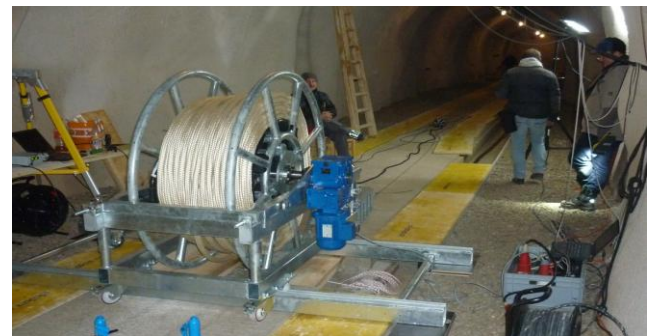
Figure 2: The winch system with LCP encased sensor cable shortly before lowering the sensor.
