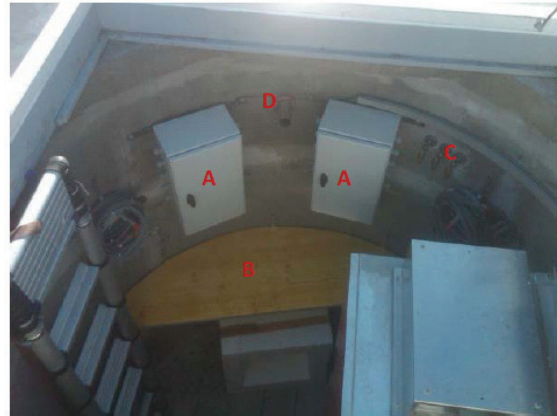
Figure 1: Enhancement of the equipment vaults: A: Signal & power switch boards; B: Equipment shelf; C: Acoustic inputs; D: GPS cables entrance.
