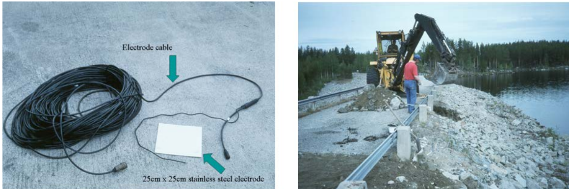
Fig. 1: Design of electrodes used for permanent installations for geoelectrical monitoring and photo from field installation in progress on Hällby embankment dam 1996.
