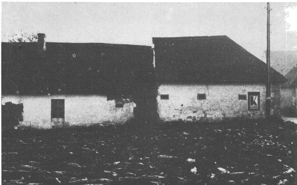
Fig. 4: Damaged building on the Diendorf Fault (in the village of Platt)
