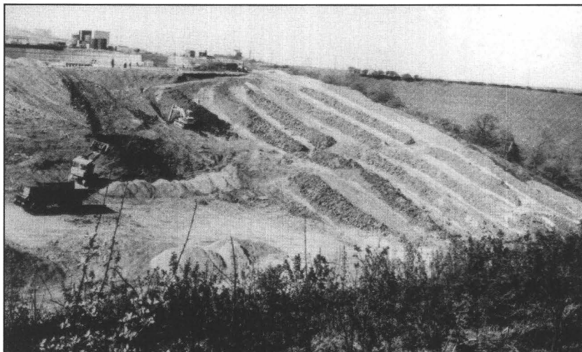
Fig. 32: Trench and counterfort drains under construction at Boulby, Yorkshire (acknowledgements to Imperial Chemical Industries Ltd., Agricultural Division, and to Cleveland Potash Ltd.).
