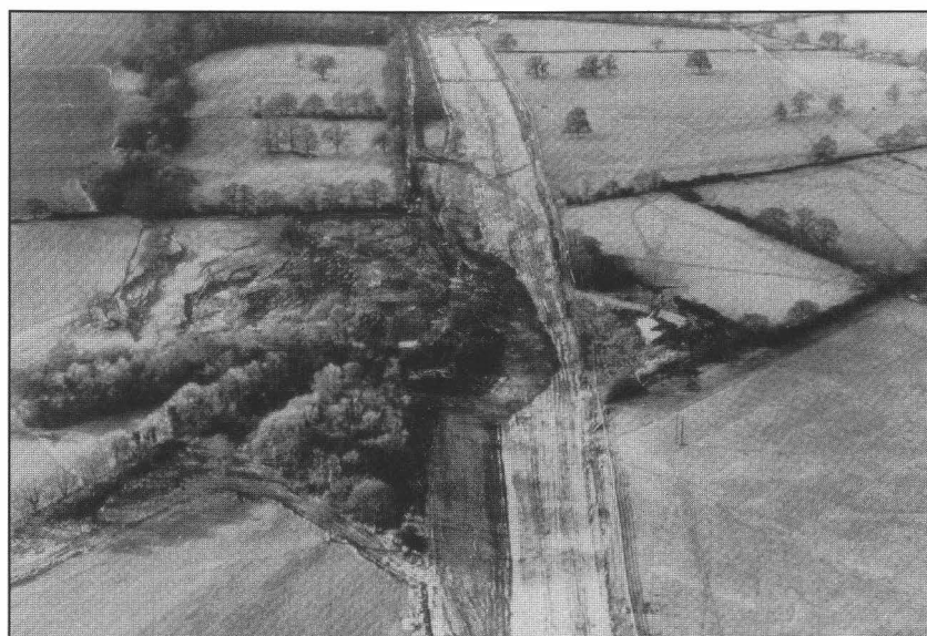
Fig. 9: Landslides into the cutting for the M4 motorway (during construction), near Swindon.
