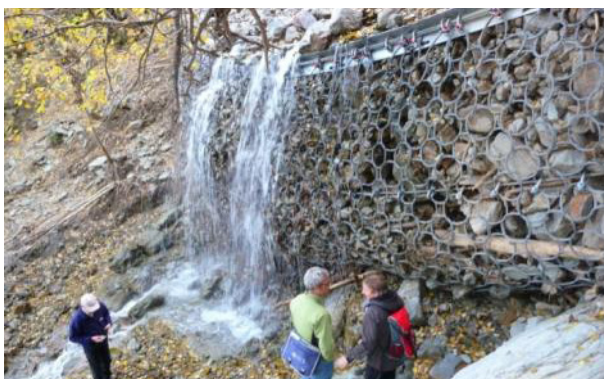
Figure 4 – Excursion site Portainé torrent with completely filled debris flow protection fences
