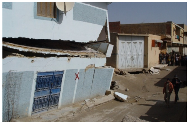
Fig. 3, Damage caused by sinkhole collapse in the Cherea town center
