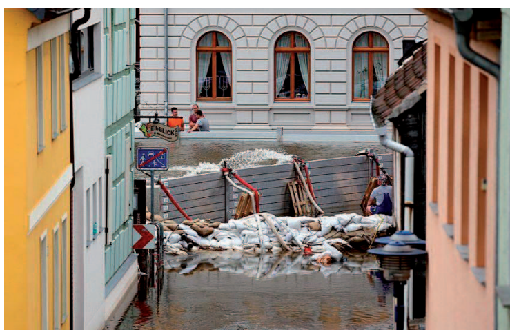
Figure 4 . Facilities for fighting floods in urban conditions
