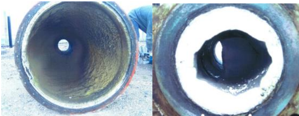
Figure 66: Pipe scaling at Soultz EGS research facility (Muller et al., 2007).
