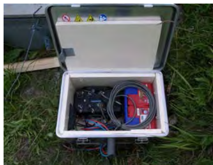
Figure 3.2: The metal box containing the electronic equipment and the 12V battery.
